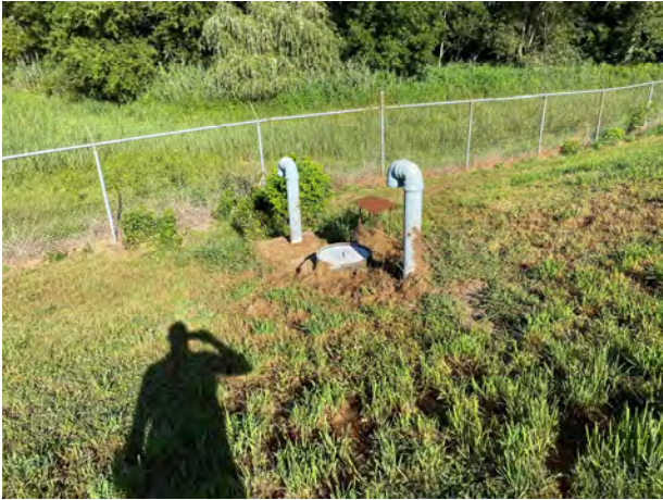
Central Byron Aeration Structure, Manhole, and Vents
