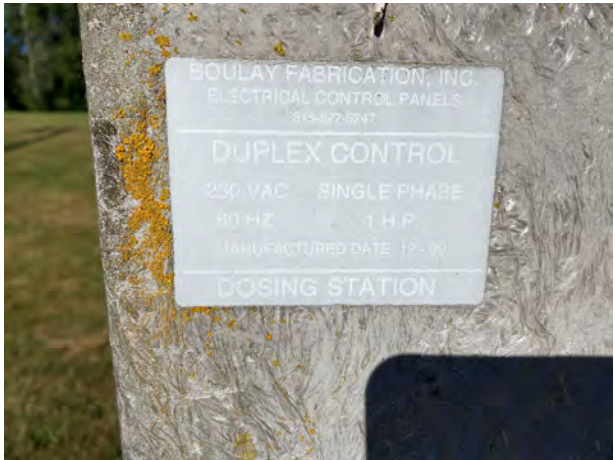
Central Byron Dosing Station
