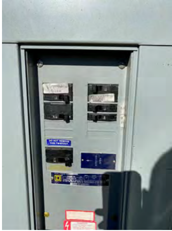
Central Byron Pump Station Controls
