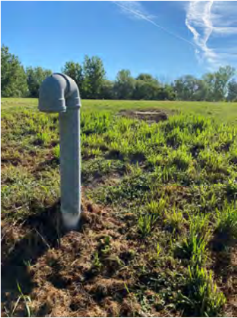
Central Byron Effluent Observation MH and Vent
