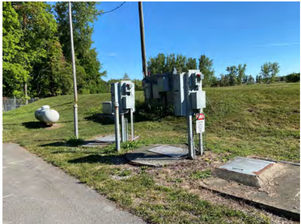
South Byron Septic Tank, Pump Station, Etc.
